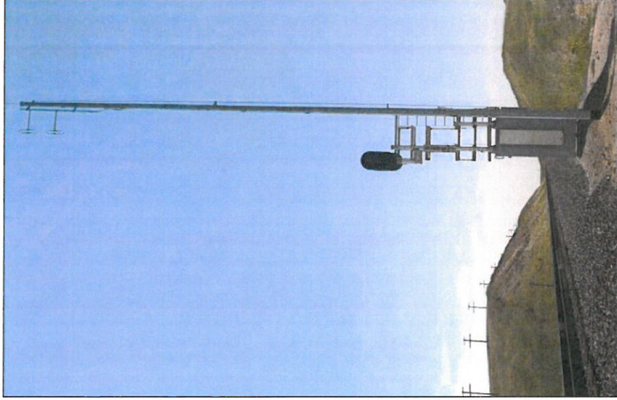
Standard PTC pole and associated equipment for UP.
