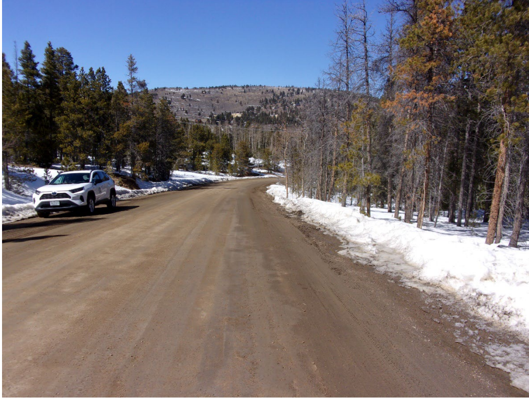
Virginia Canyon Road Conditions looking North.
